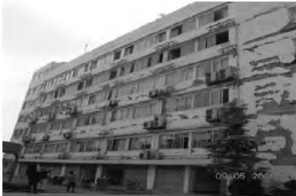
Horizontal cracks of infilled walls.
